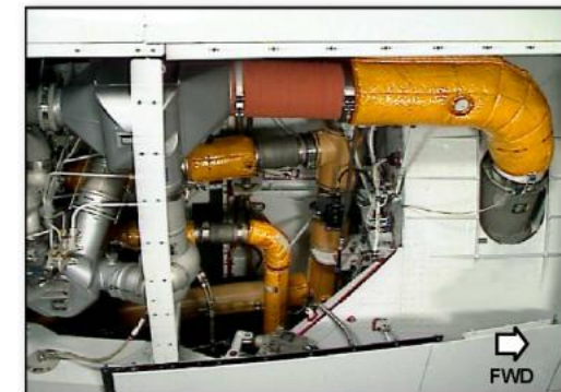
AIR CONDITIONING COMPARTMENT
