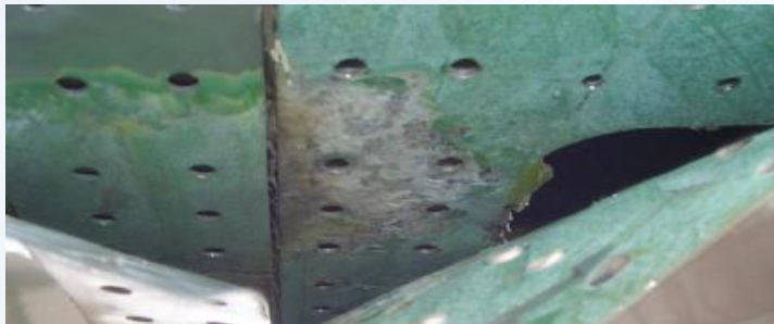
盖板缝隙处的腐蚀
